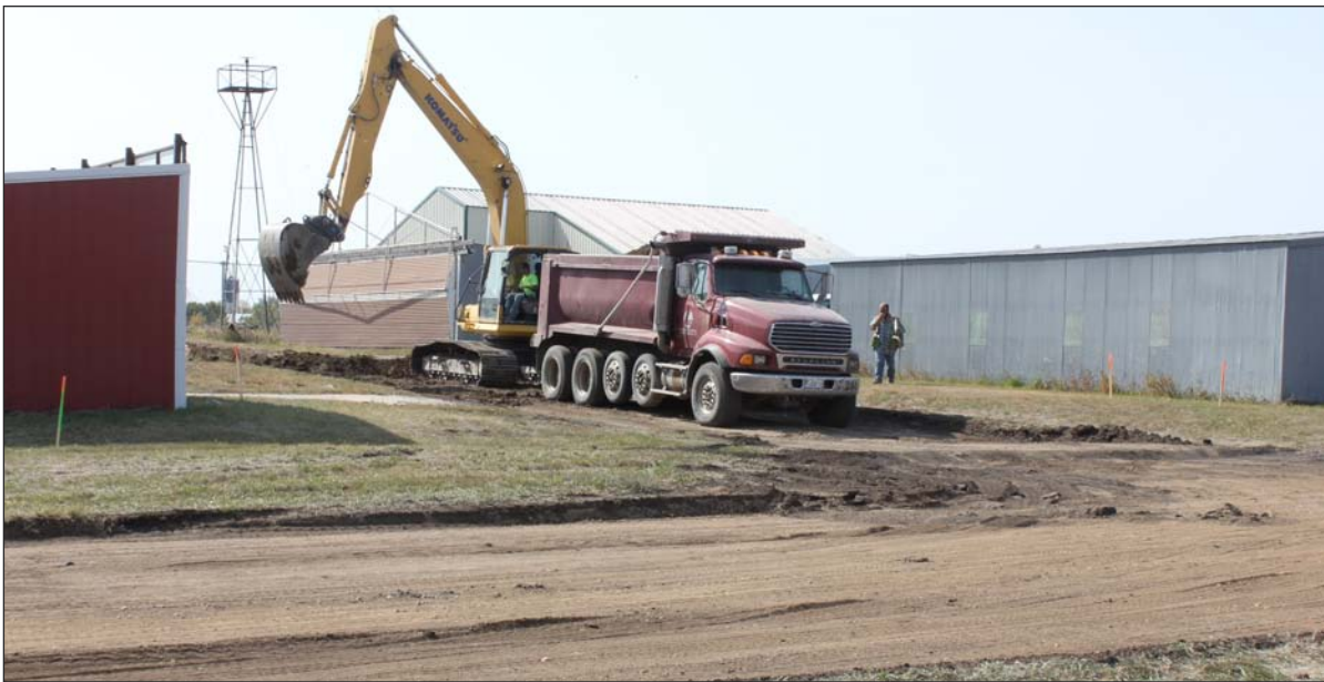
City maintenance chief Jerod Raethz said at the city council meeting on Monday that the Airport taxi lane project was proceeding well and that he expected work to be completed within the next two weeks. City Finance Officer Lisa Raethz told the Faulk County Record that the Total Cost: of the project is $315,000, the Federal Share: 90% $283,500, the State Share: 8% $25,200 and the Local Share: 2% $6,300.
