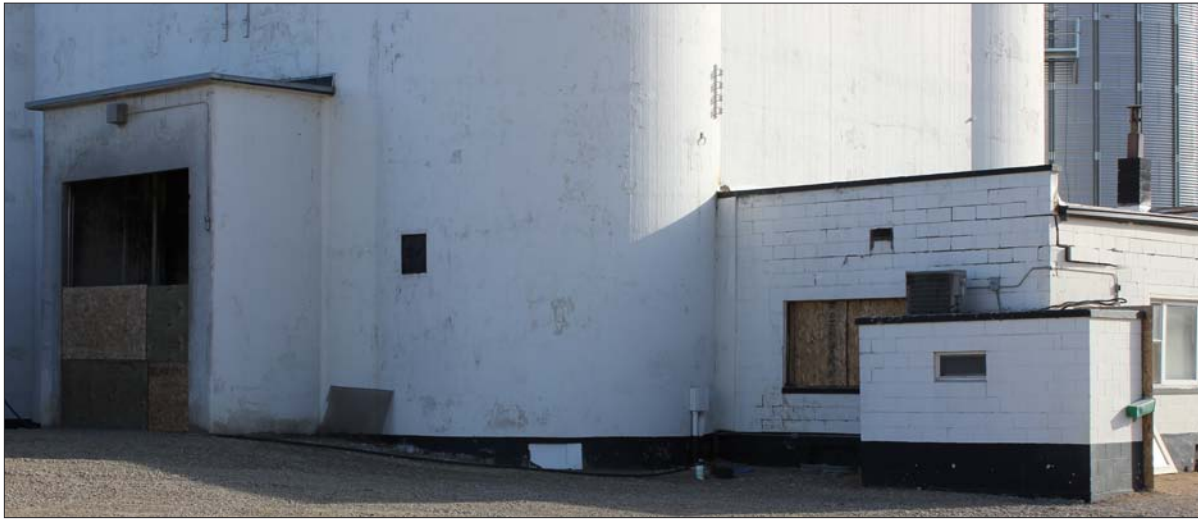
The extent of the damage to North Central Farmers Elevator following Friday's explosion will not be determined until an insurance investigation is completed. Damage viewed here shows where a window was blown out and structural damage along the roof line. Below also shows upper wall damage on the west side of the office.
