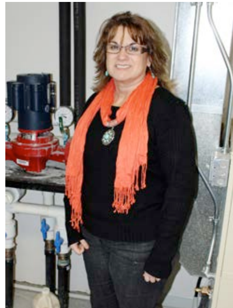
From top: Jason Ferguson at the Faulk County Courthouse and Sandy Bowar at the USDA Service Center both say their geothermal systems require little adjusting, no matter the season.
